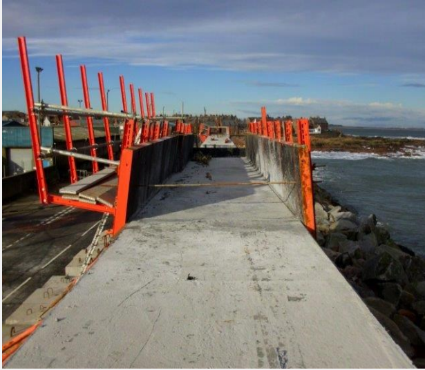
Shutter during construction. The road to the left the sea to the right
